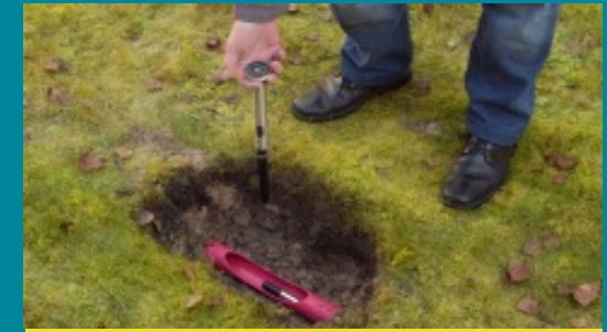
The sonde can be positioned very precisely and it helps to avoid extensive trenches.
